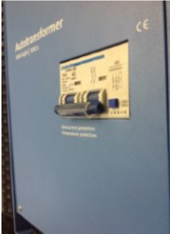
The MCB for over current and temperature protection and ON/OFF switch
