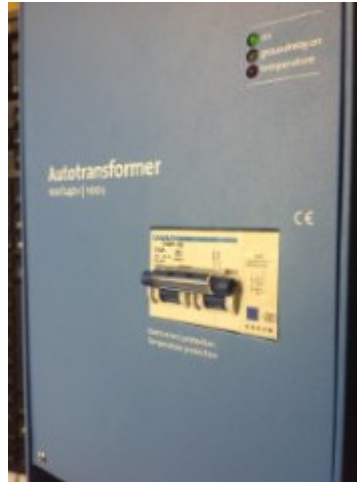
The Autotransformer is on. The green LED is on.
